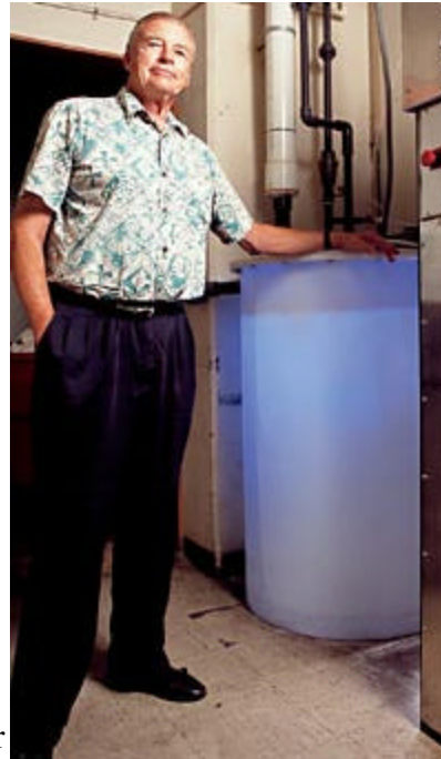
BLUE TANK GROUP: John Connors' Ozone Industries Inc. engineers and sells water treatment systems such as this one in the Waikiki Beachcomber Hotel's laundry room. Photo: Jimmy Forrest
